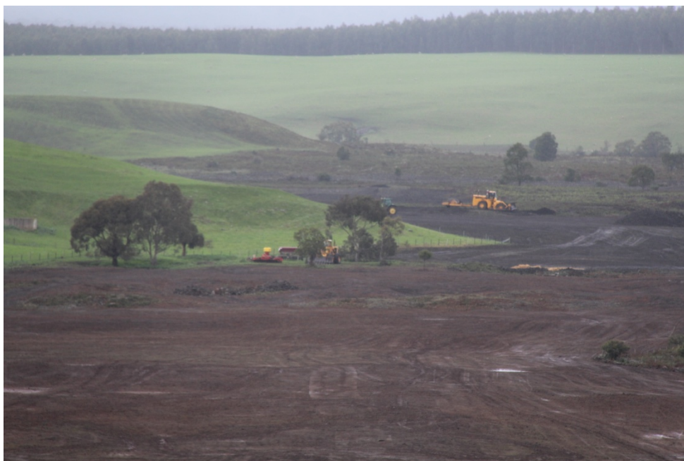
Figure 1. Harman's Valley rock crushing proceeding in July 2016. Photo taken from the Port Fairy-Hamilton Road Lookout looking east toward Mt Napier.
